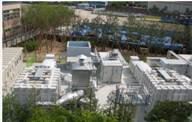
[ SH District Energy Site Sanggye area: 2.8MW ]
