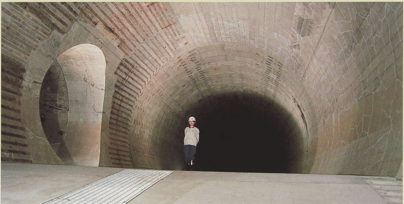
Zenpukuji River intake facility connecting duct joint points of the Stage 1 tunnel
