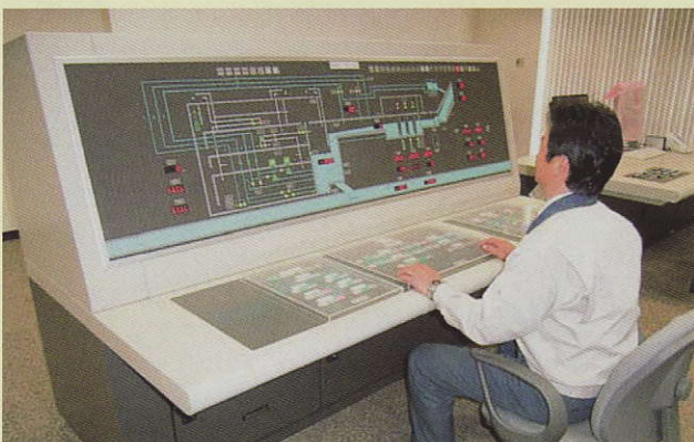
Central monitor and control board of Zenpukuji River intake facility
