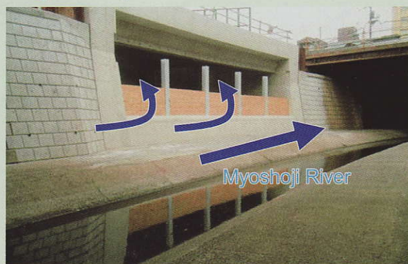
Myoshoji River Intake Facility and Intakes
